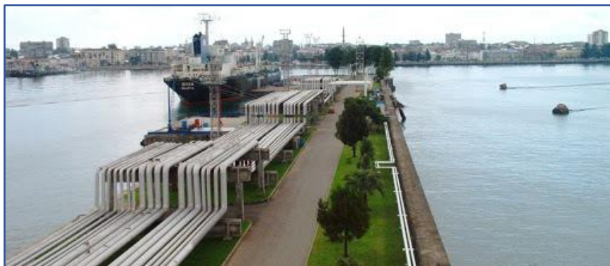
Fig. 1. Batumi oil terminal.
